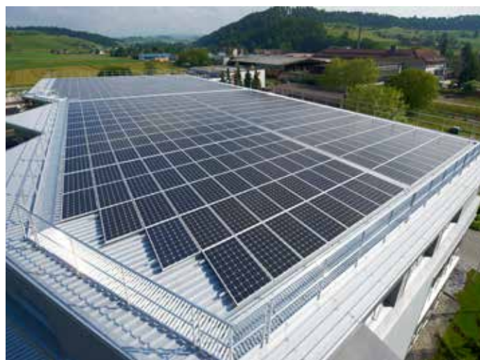
Photovoltaic system with a performance of 162 kWh.
