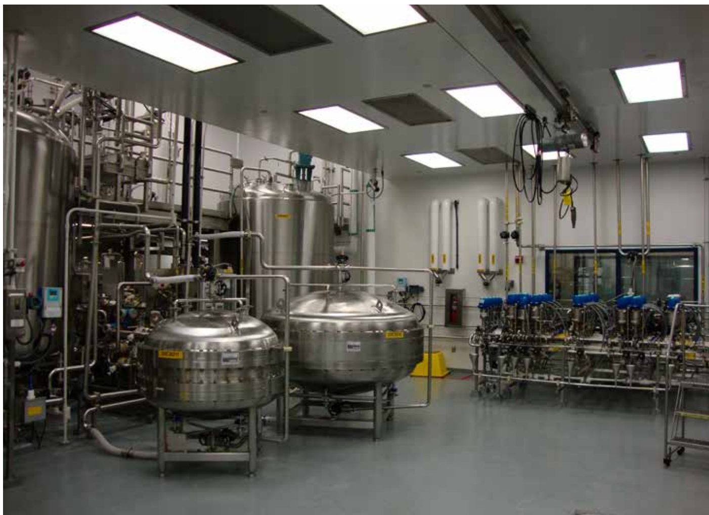
Modern immunoglobulin purification facility
